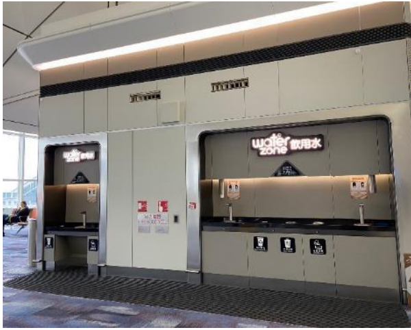
Water Zones installed inside terminal and concourse at HKIA
